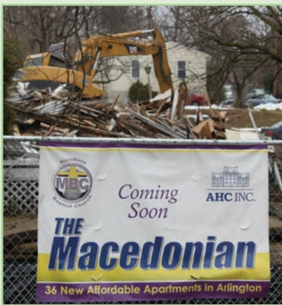
In February, bulldozers prepared the site for construction of 36 new affordable apartments in Arlington's Nauck neighborhood. AHC is partnering with Macedonia Baptist Church on the project.
